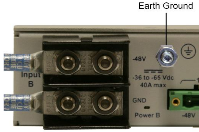
Input Feed B and the Grounding Lug for the RPS AB6
