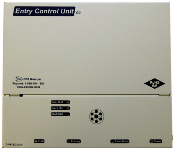
The ECU LAN provides comprehensive access management for a single door
